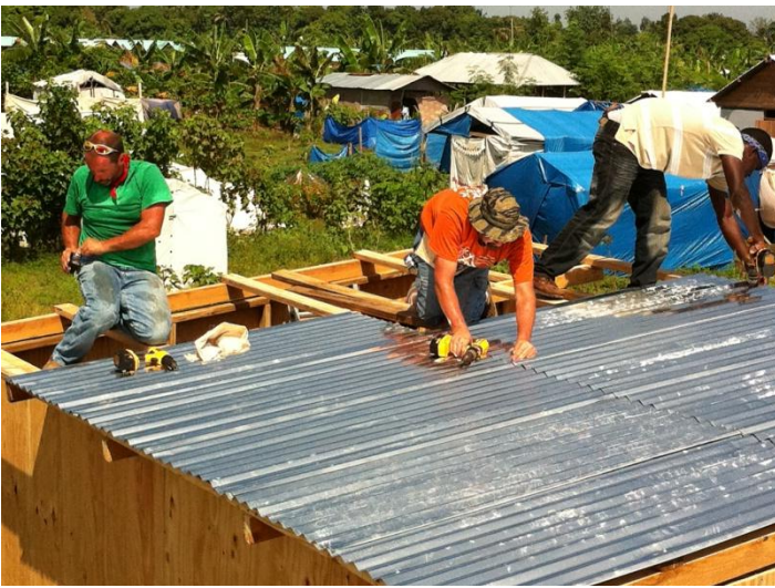
Again, the heat was unbearable at times especially when completing this type of work. Luckily, we had good tools that expedited this portion of the project.
